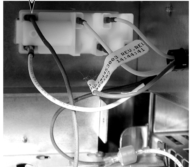
Ignition Switch Wire Connector At Spark Module
