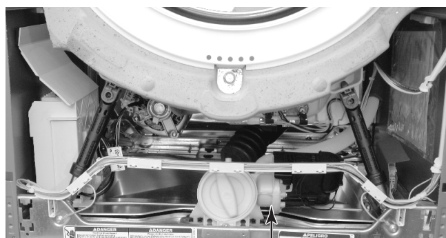
Drain Pump Assembly
